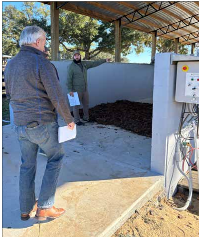
Ron Losasso and Steve Talbott inspecting first load of stable waste into the Earth Flow composter.
